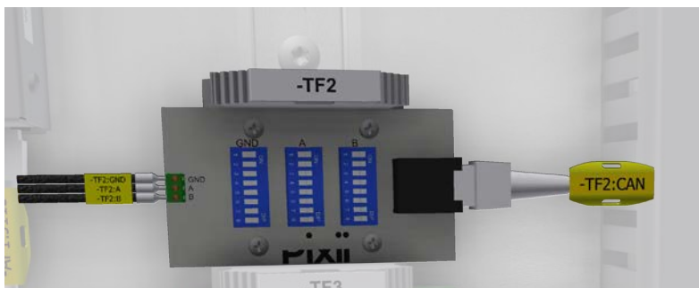
Figure 4.28 Battery Com converter (-TF2)
