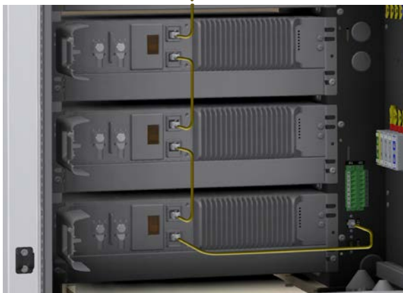
Figure 4.26 Battery communication cables
